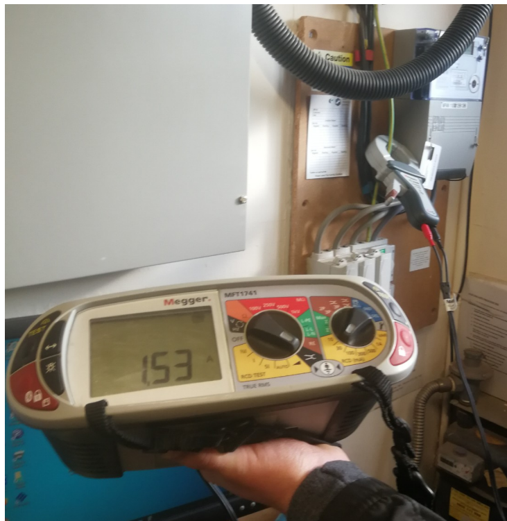
Illustration 3: Measurement on an Earth Conductor of current from a shared water system in a multi-occupancy brick building with multiple TN-C-S supplies
