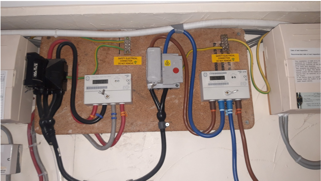
Illustration 2: 2 TN-C-S supplies installed in a common switch-room. Thanks to M. Harris
