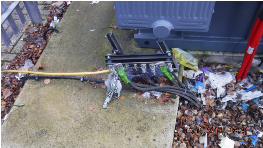
Illustration 1: Earthing systems don't always get looked after well, even if they've been installed correctly in the first place.
